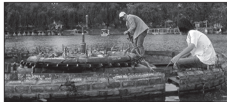
Taking measurements of the existing fountain facilities in the middle of Burnham Lake.
